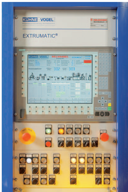
Standardised process control and visualisation of an extrusion system at our Windsbach factory.
